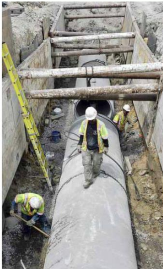
Baltimore Water Pipe
